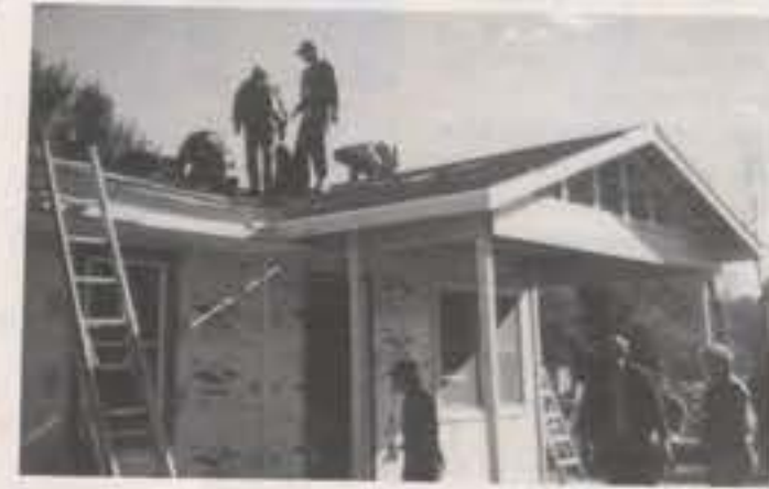
Volunteers under the leadership of Steve Eveleigh and Dan Leary work on the Kingsley home. Steve is chairman of the HFH-GTR Building Committee.
