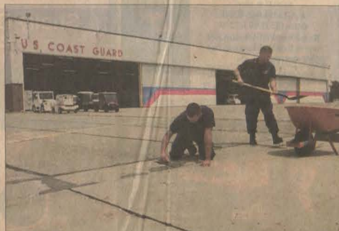
Fireman Eugene Sapelli, left, and Chief Petty Officer Dale Ashley repair cracks in the tarmac outside the hangar at Coast Guard Air Station Traverse City.
